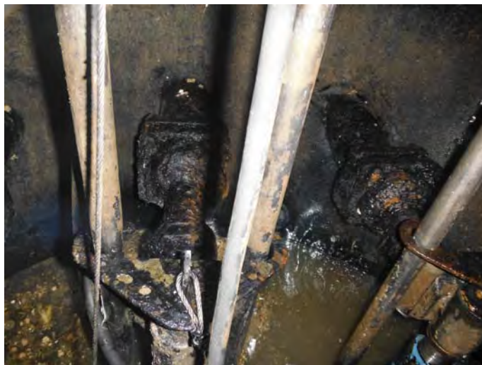
SLS #7 Wetwell Piping
