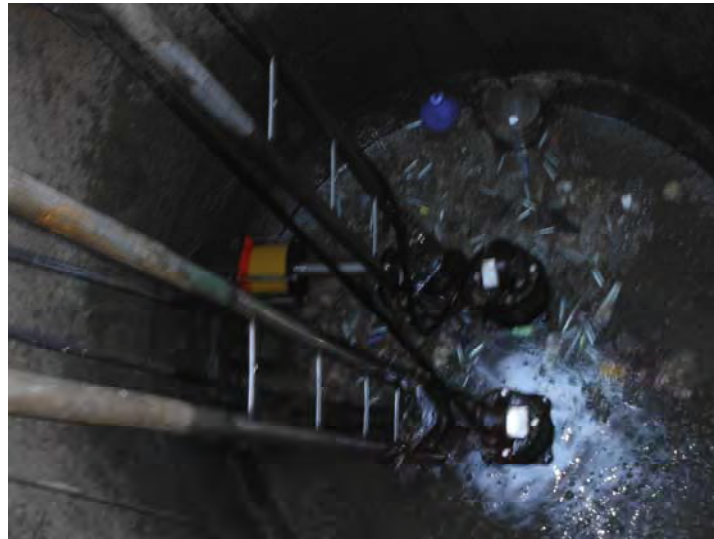
SLS #9 Wetwell Piping
