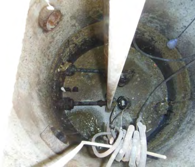
SLS #8 Wetwell Piping
